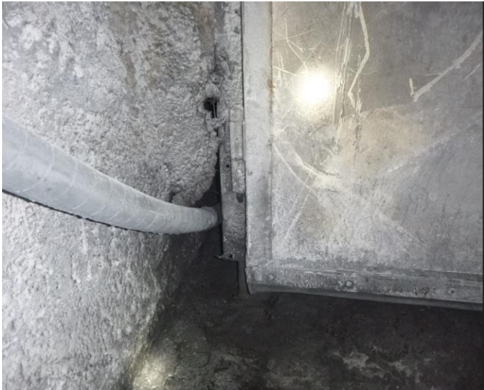
Leakage path around door
