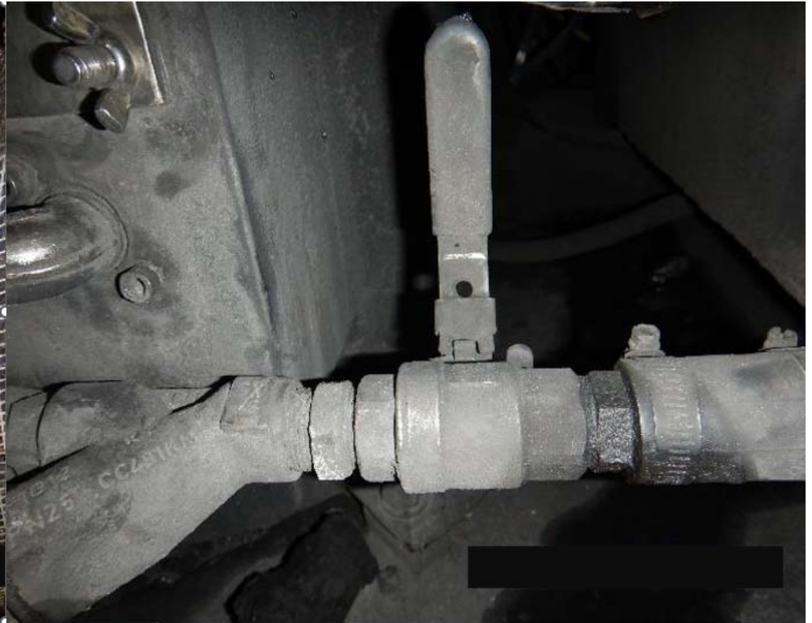
Scrubber Valve Off
