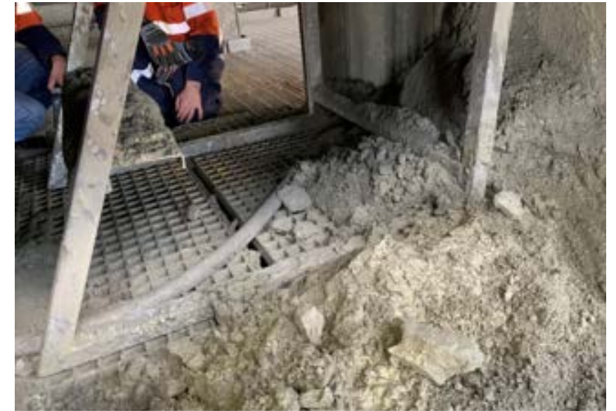
Inside the chamber after the incident
