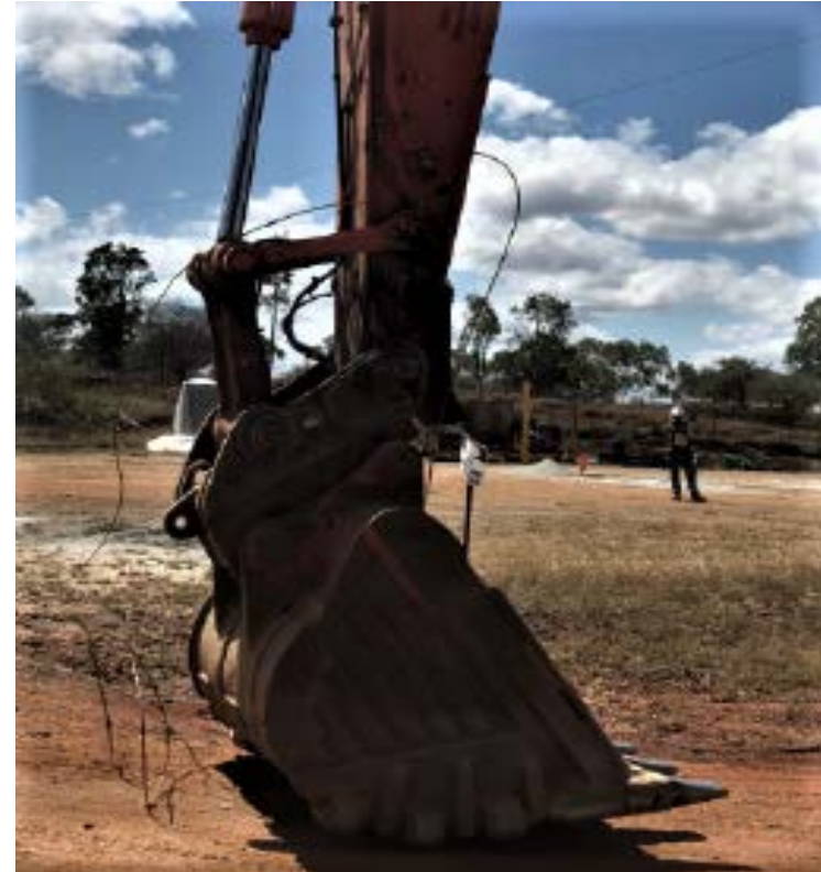
Conductor entangled around excavator boom
