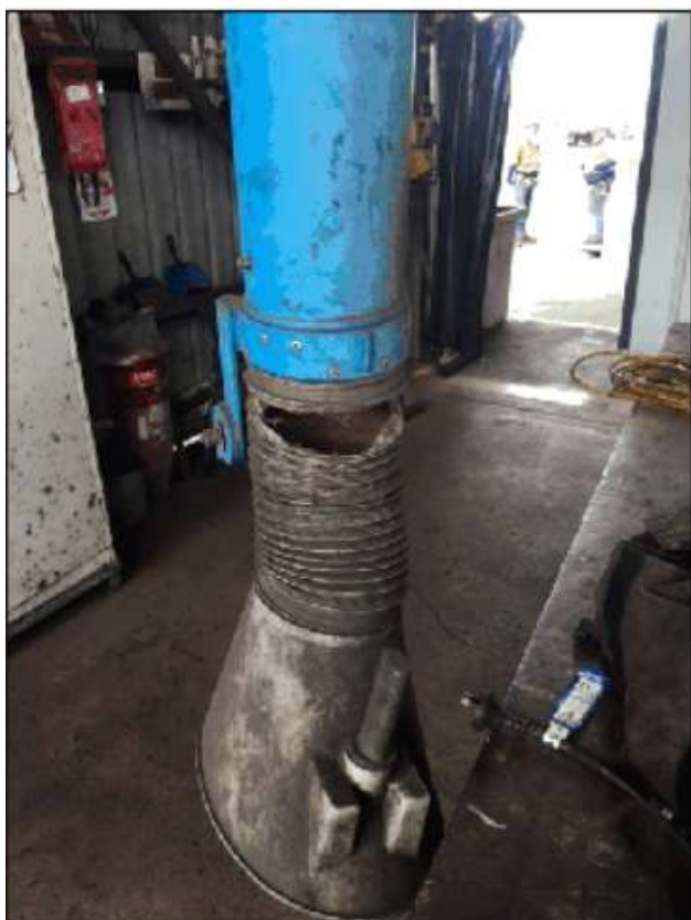
Figure A7: Poorly maintained LEV systems
