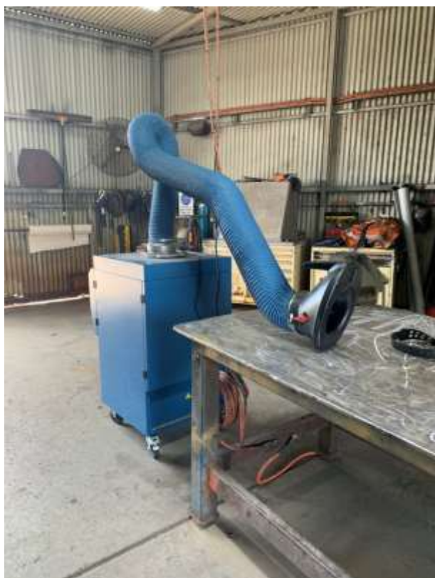
Figure A3: Local exhaust ventilation being used and well maintained
