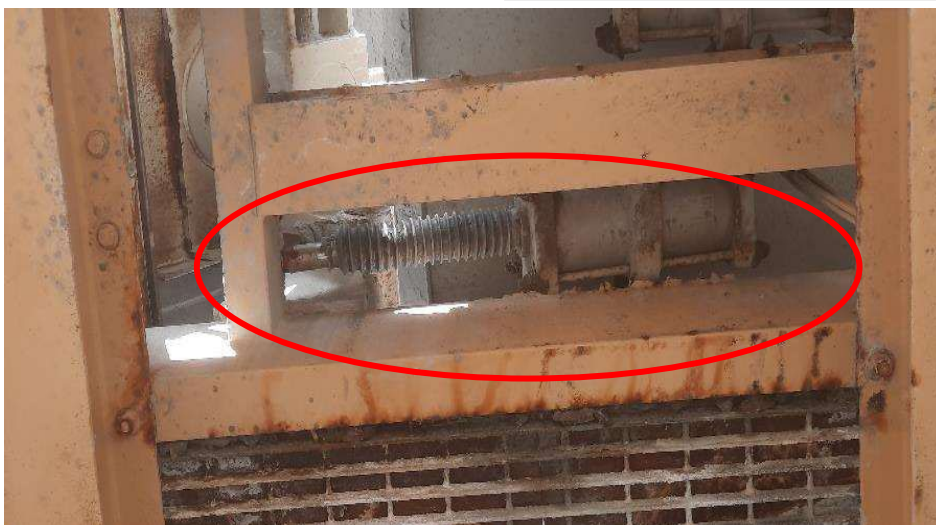
Fig 1 Failed pneumatic ram
