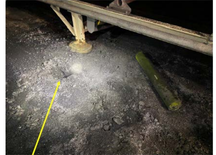
Impact mark in ground beside overland conveyor transfer belt
