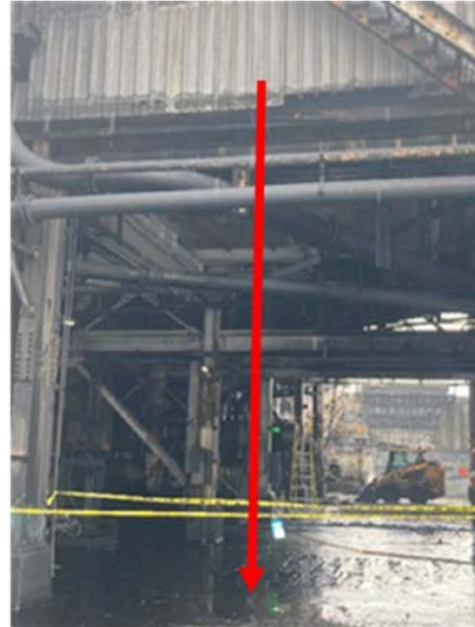
Z purling's and crowbar fell 6m est.
