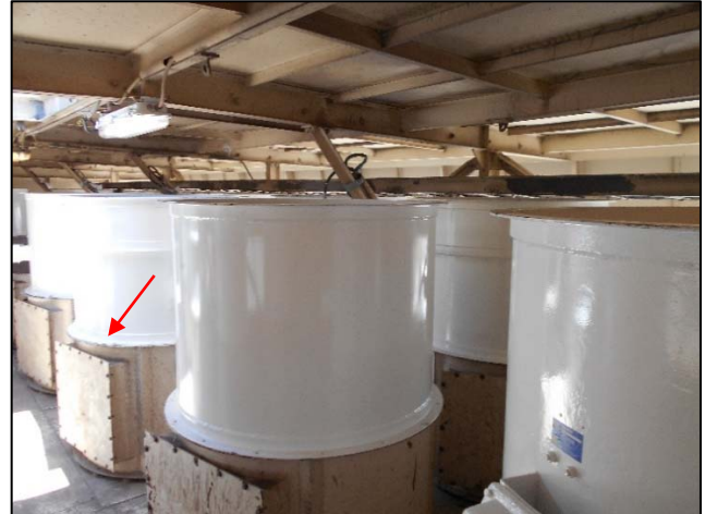
Photo 19: Access hatch to dynavanes for cleaning
