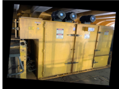
Prevent entry into enclosure
