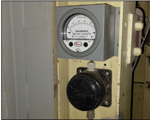
Photo 6: Pressure Monitoring System
