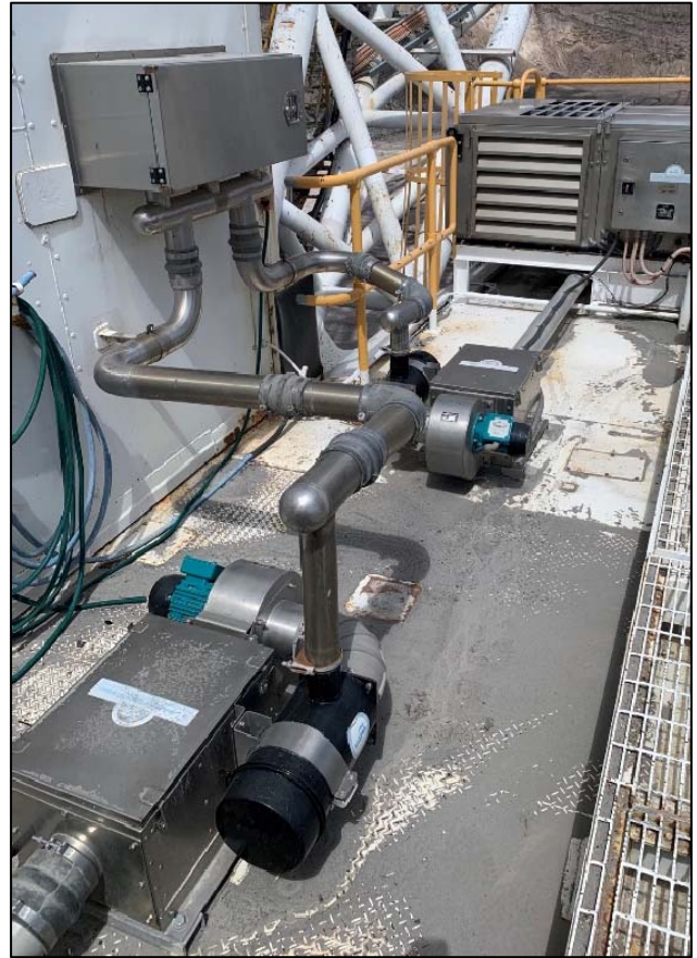
Photo 22: HEPA filtration system for dragline operator Cab
