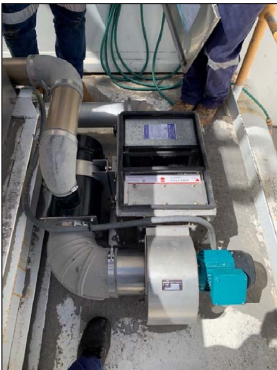
Photo 8: HEPA Filtration of Dragline House Air
