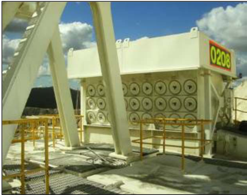
Photo 14: Cartridge / Baghouse Technology on Shovel (10)
